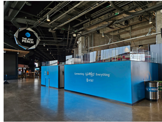
Sightline Commercial Solutions custom engineered and installed 775 linear feet of glass guardrail.
