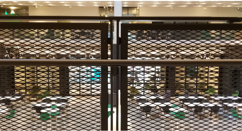
Steel toe kick plate added below the guardrail on overlooks and landings prevents smaller objects from falling over the edge.
