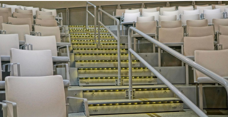
LED lighting integrated into stair units mark aisles and ensures audience members can see stair edges.
