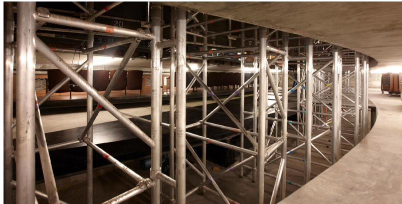
A custom beam and support structure accommodates for an increased load rating.
