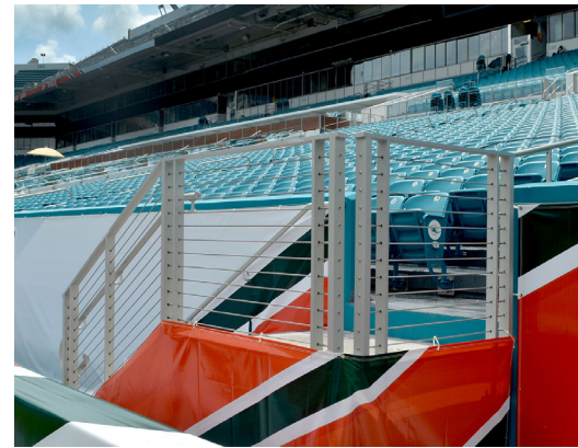
Cable railing used at front of bowl, ADA seating areas and stairways down to field level.
