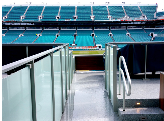
Custom post supported glass railing attached via top and fascia mount.
