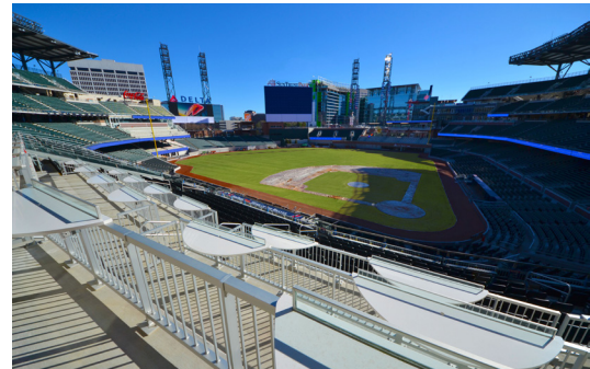
Custom quarter round aluminum support plate and gussets for the solid surface tops to sit on.
