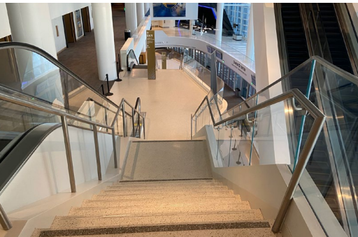
Aluminum handrail attached to the glass infill to safely guide patrons.
