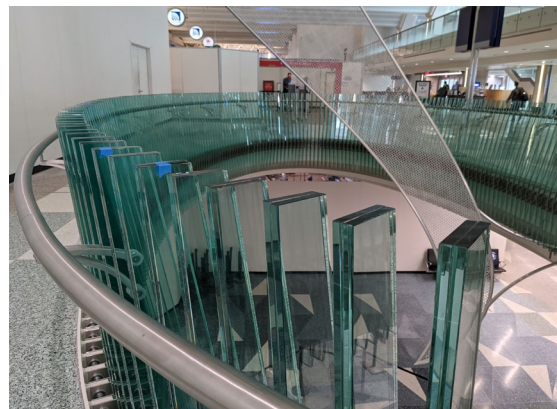
Glass fin railing panels were positioned vertically around the second story overlook.
