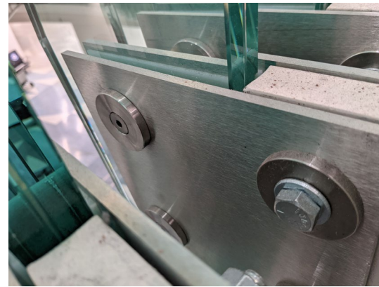
The clear glass fins and knife plates are expertly fit using steel connection pieces that bridge the individual panels to the bottom of the railing system.
