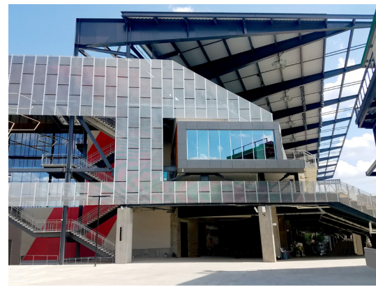
A 6,320-square-foot custom perforated panel wall surrounds the entire north face of the East Building.
