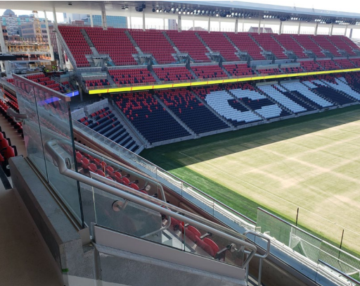
Our team engineered and installed more than 17,000 linear feet of custom railing.
