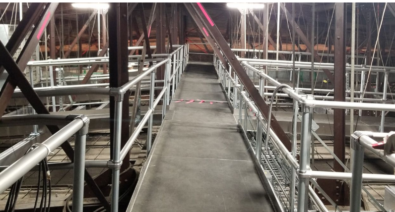
We developed a catwalk-inspired access platform system positioned 80 feet above the main floor of the theater.
