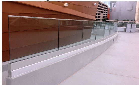
Back side of the custom LED lit C-channel base shoe glass railing system.
