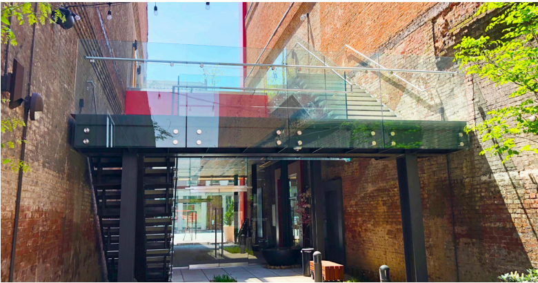
Point railing is used on both sides of the bridge to provide a safe and stylish walkway to the exterior courtyard.
