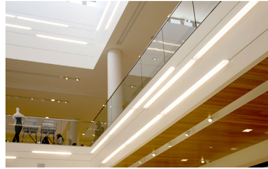
Base Shoe glass railing on balcony overlook with 1/2" clear tempered glass.
