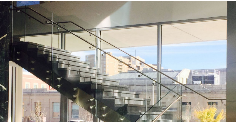
Point railing with 2 1/2" stainless steel side mounted nodes attached to metal stair stringer via drilled and tapped epoxy anchors.
