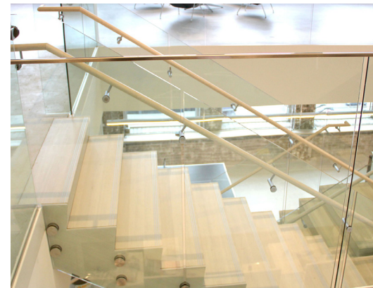
Base shoe with 1/2" glass shoe anchored to the structural slab on balcony overlooks.
