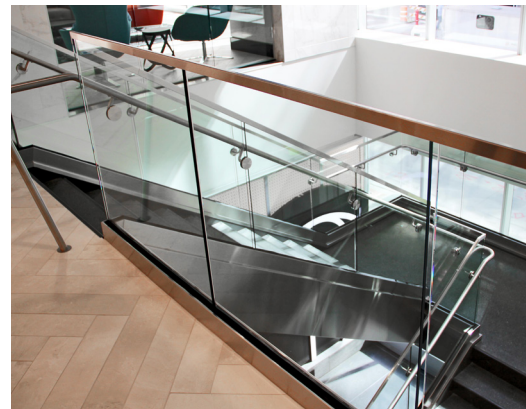
Multiple stairs and overlooks utilized the Track Rail system with glass infill allowing light to flow throughout the lobby area.
