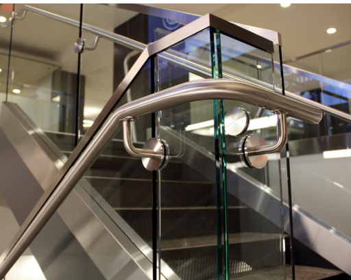
On interior stairs, stainless steel handrail was attached to 1/2" clear tempered glass with thru-glass stainless steel standoffs.
