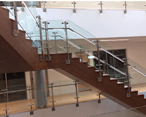
Railing posts were fascia-mounted, directly to the stair stringer.
