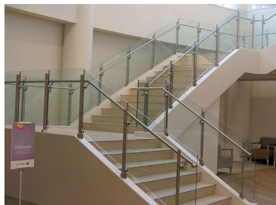
Stainless steel trapezoidal posts were welded to structural steel stair stringers at the monumental stair and finished with custom escutcheon covers.
