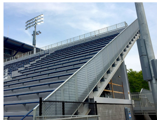
USTA's South Campus fan seating areas utilize Gridguard grated railing attached to brackets stud welded to the raker beams.
